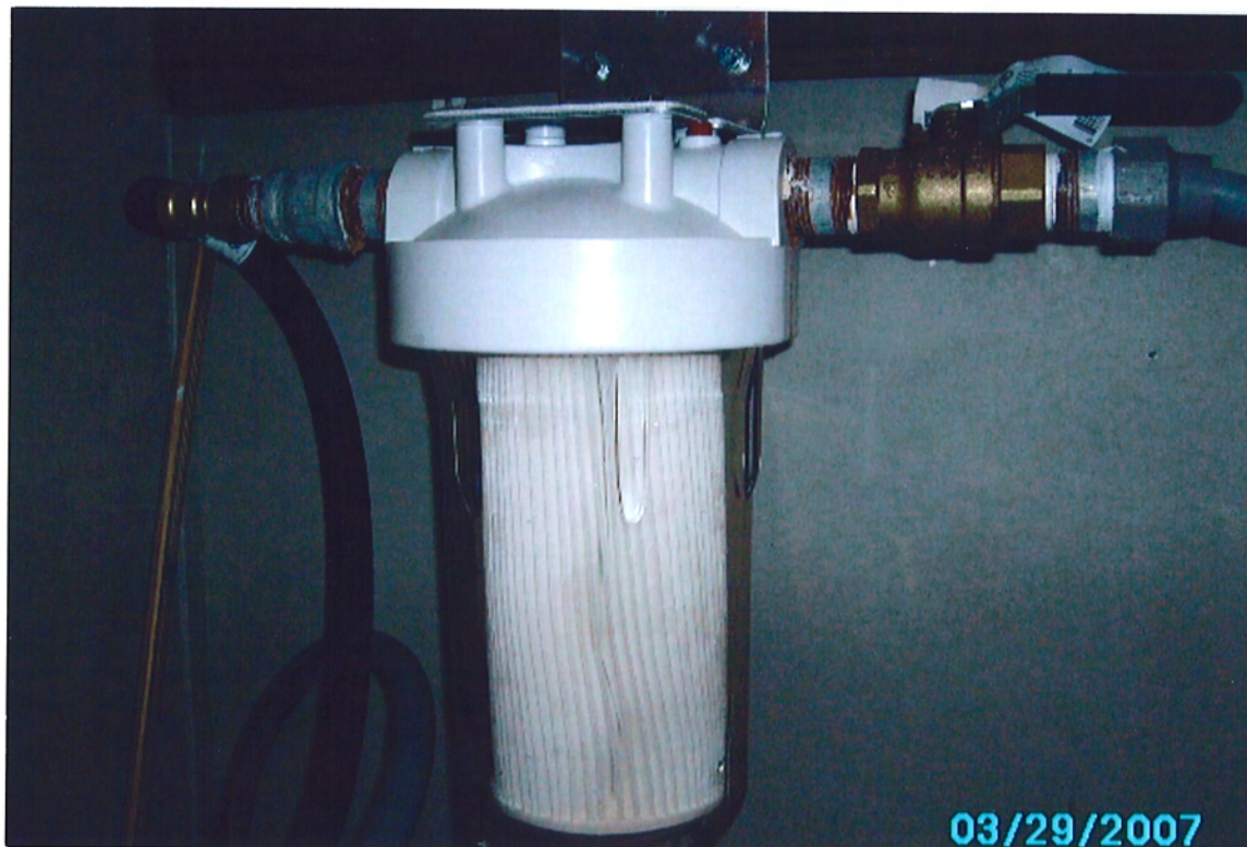
Photo 4: March 29, 2007 – New water filter installed in Complainant's home
